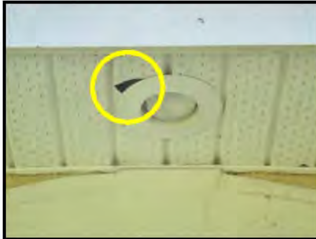
Areas of soffit need to be sealed
