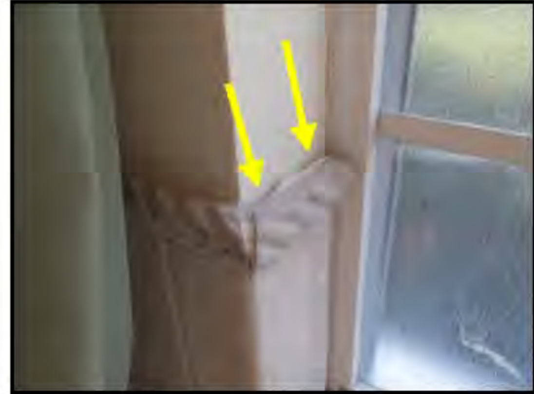
Loose tile trim noted on sides of window in Master Bathroom
