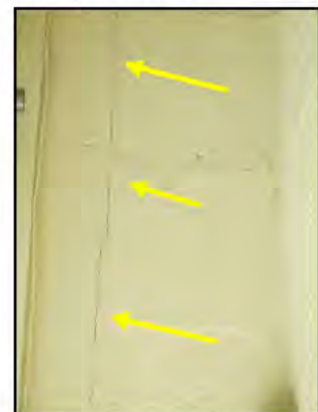
Minor settling cracks noted, No concerns at time of inspection
