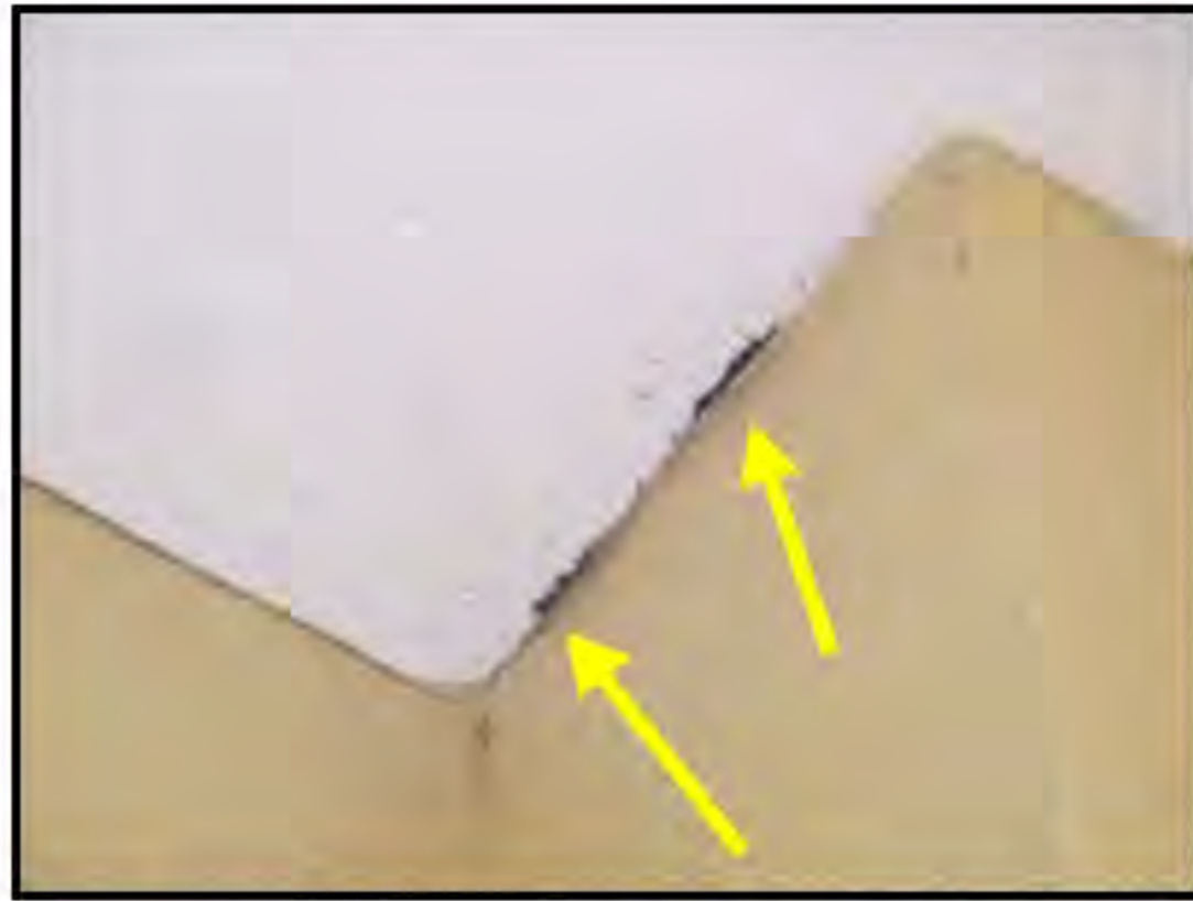
Tape joints releasing in corners of Front Entryway Ceiling
