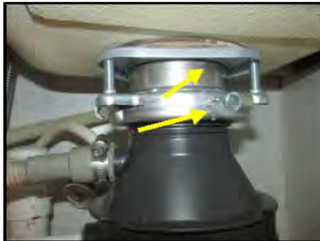
Minor water leak noted at sink connection while in use, Check seal or tighten unit
