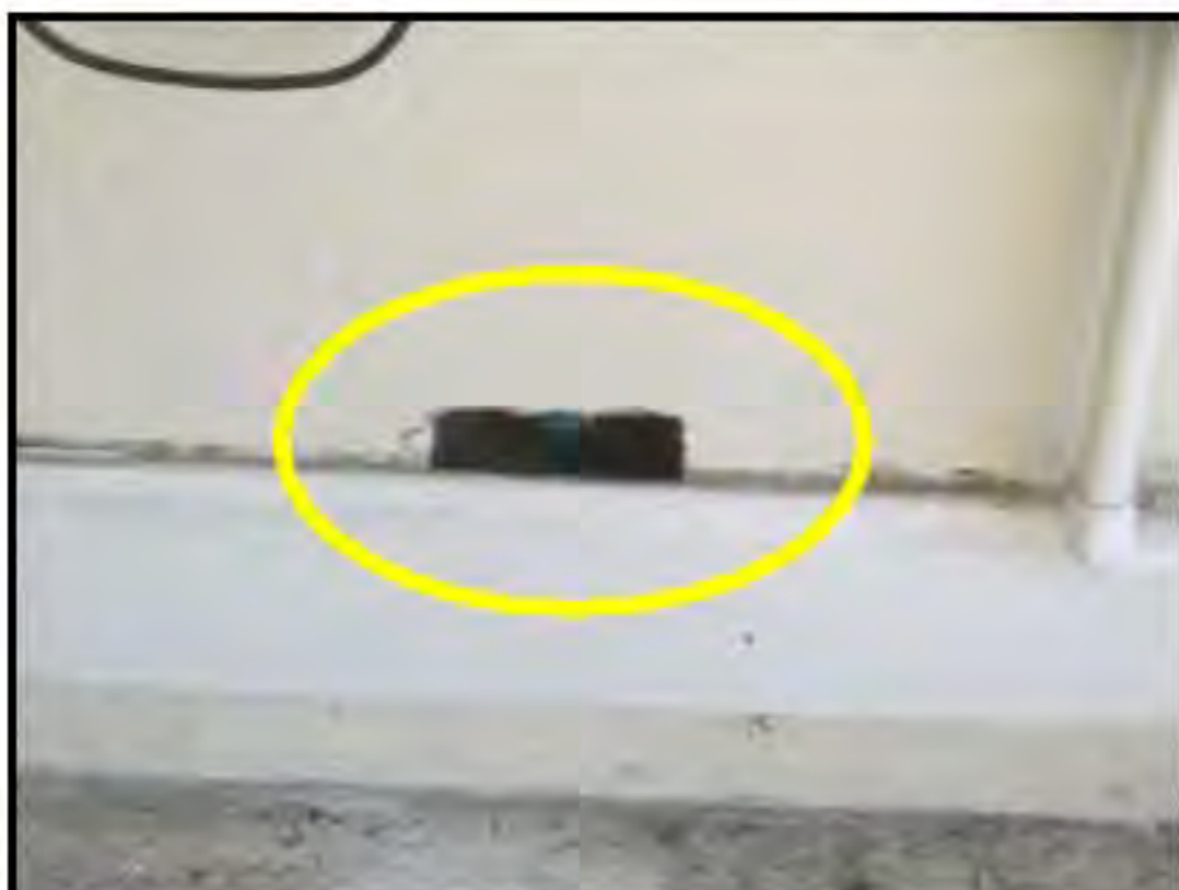
Minor holes noted in areas
