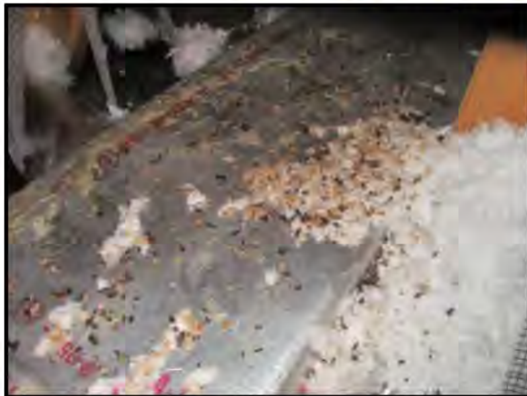
Signs of past animal/rodent activity, recommend sealing all holes/spaces in soffit to prevent access
