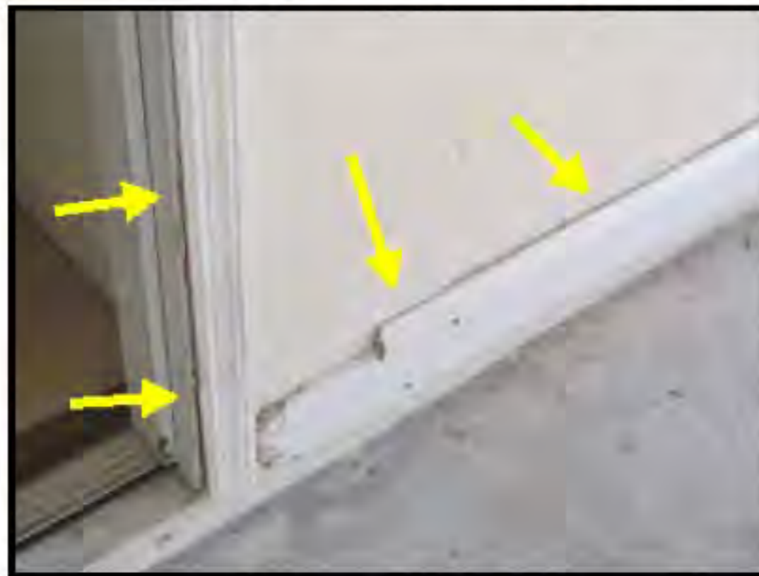
Garage Interior Door jamb trim and base loose
