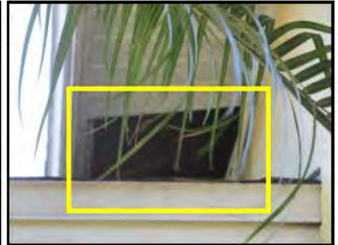
Some soffit panels missing
