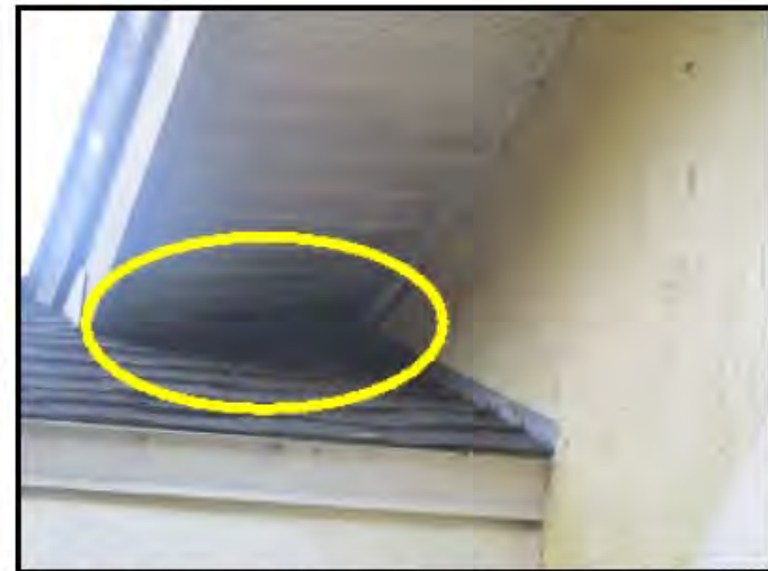
Some soffit panels missing
