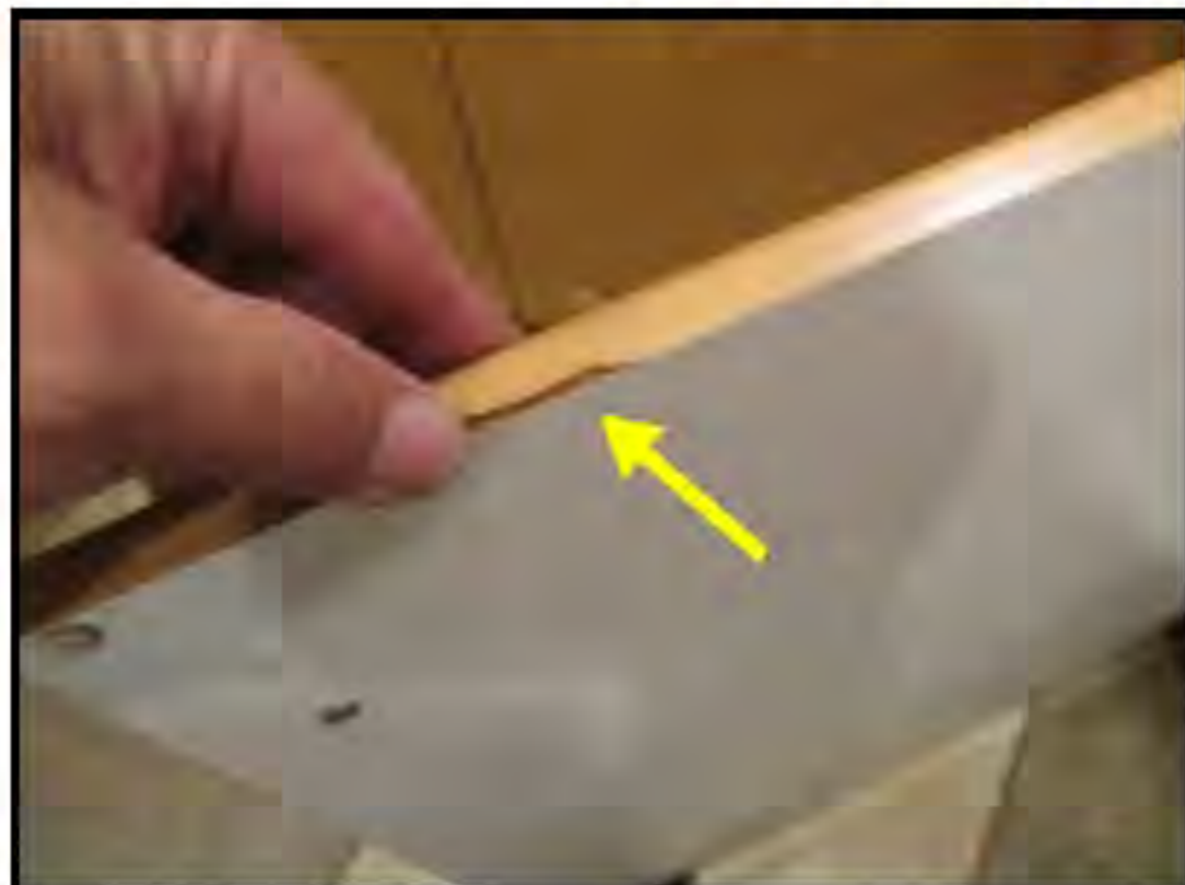
Cabinet door edges de-laminating in areas
