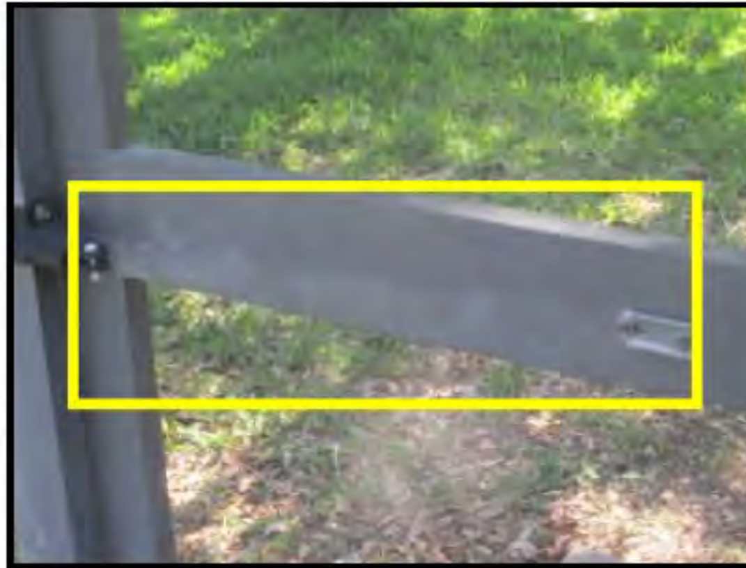
Closer on side Screen Door missing
