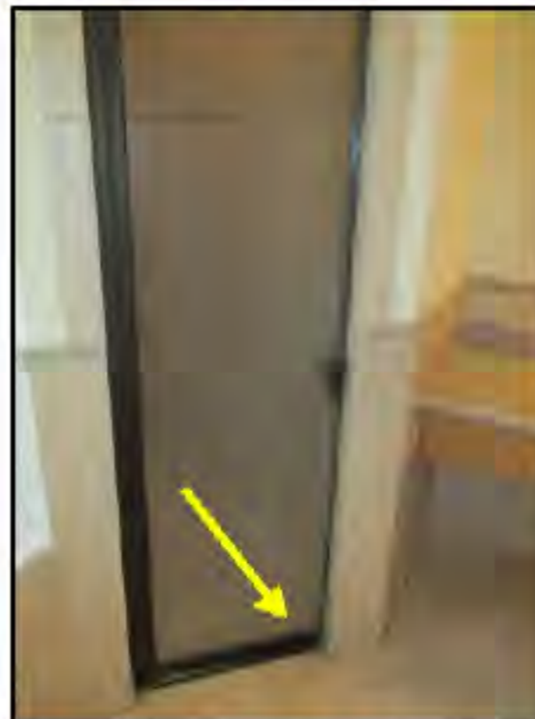
Shower Door in Master Bathroom binds/sticks at bottom, Needs adjustment
