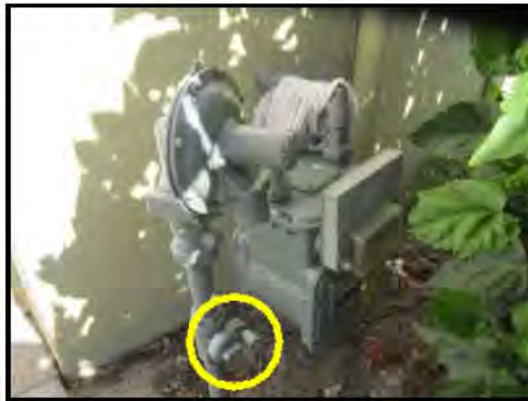
Gas was Off at time of inspection, unable to fully inspect gas systems in home
