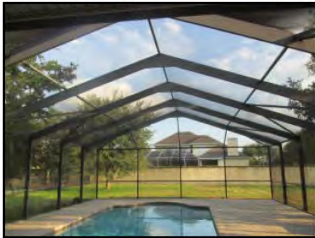
Appears to be sound structure and in satisfactory condition at time of inspection
