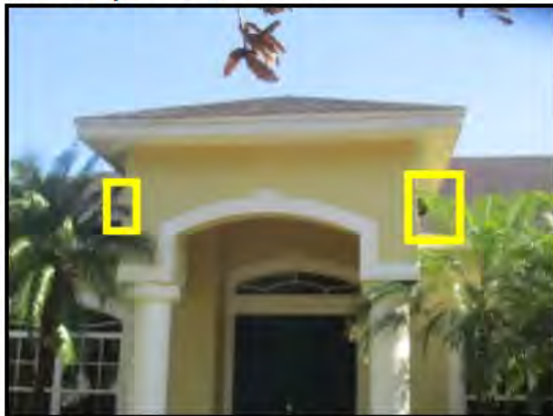
Some soffit panels missing
