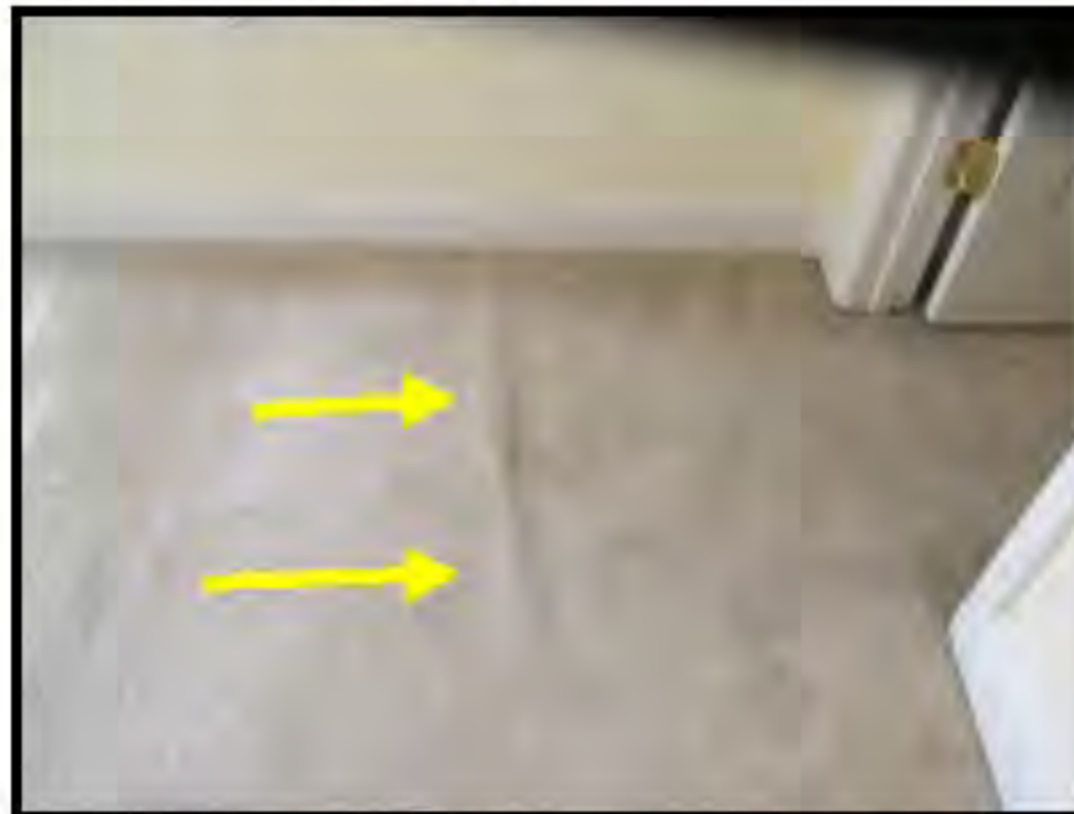
Carpet needs restretching
