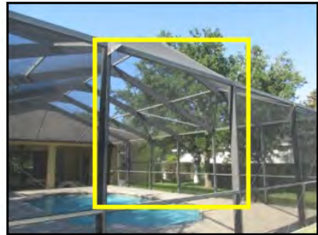
Back screen panel missing at time of inspection
