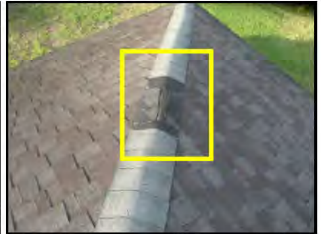
3 ft of Ridge Cap missing on front left side of home
