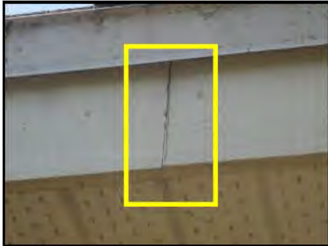
Fascia is wood, Recommend maintaining proper maintenance to further protect areas
