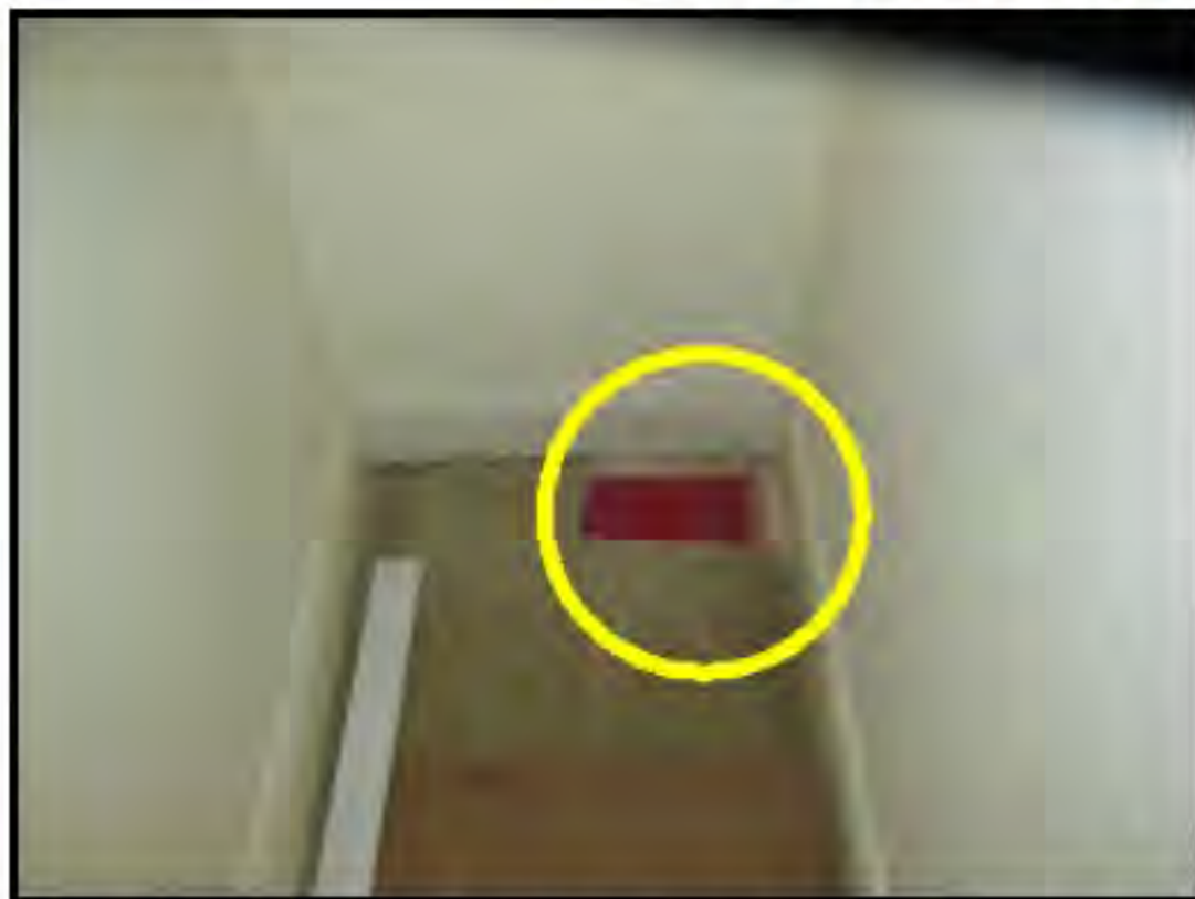
Carpet cut/missing in corners of both back bedroom closets
