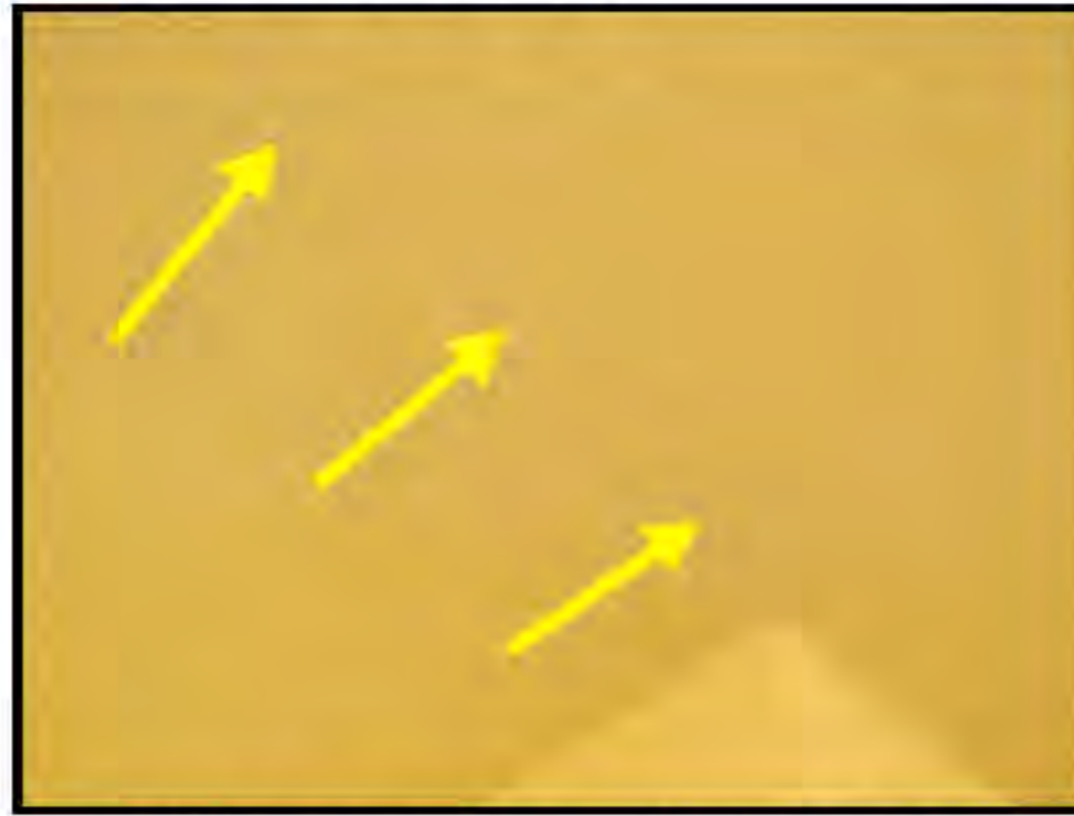
Settling cracks noted in areas
