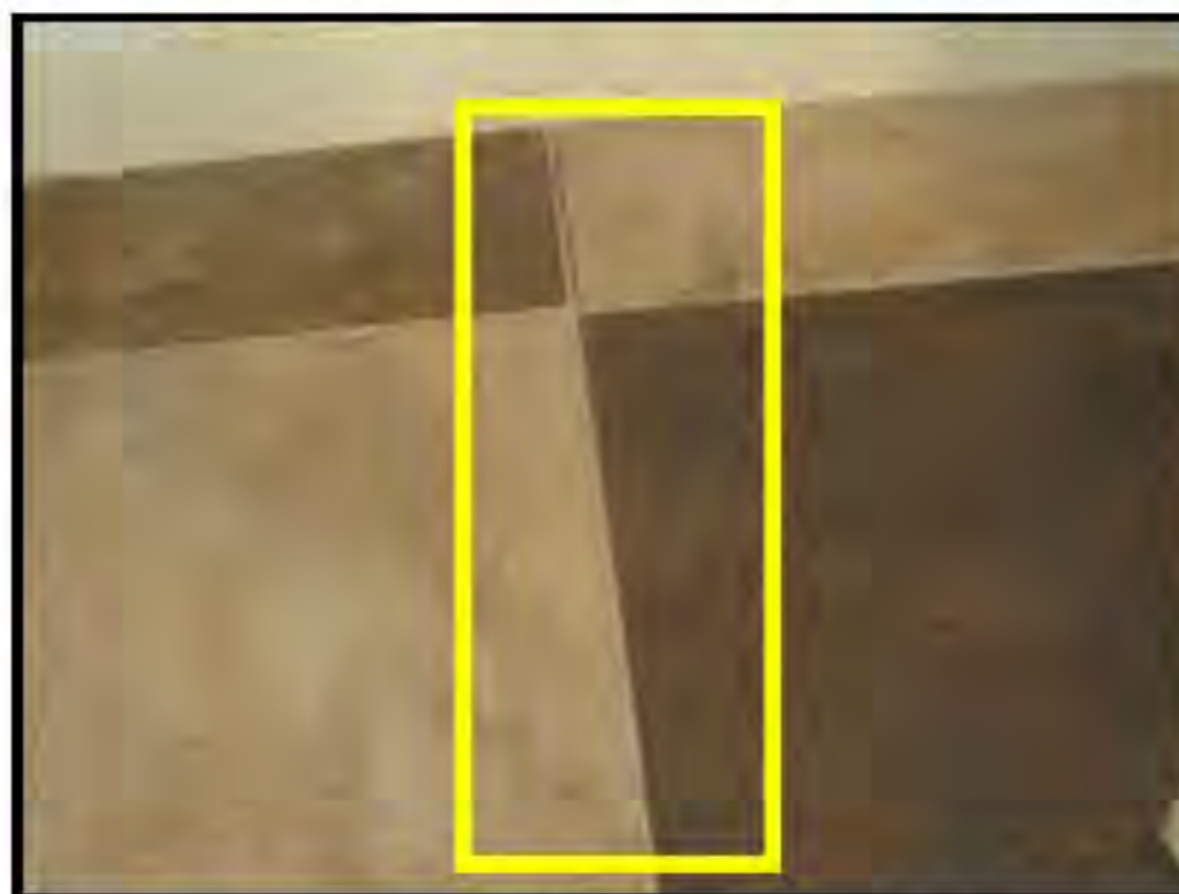
Tile grout cracks noted in Hall Closet next to Utility Room
