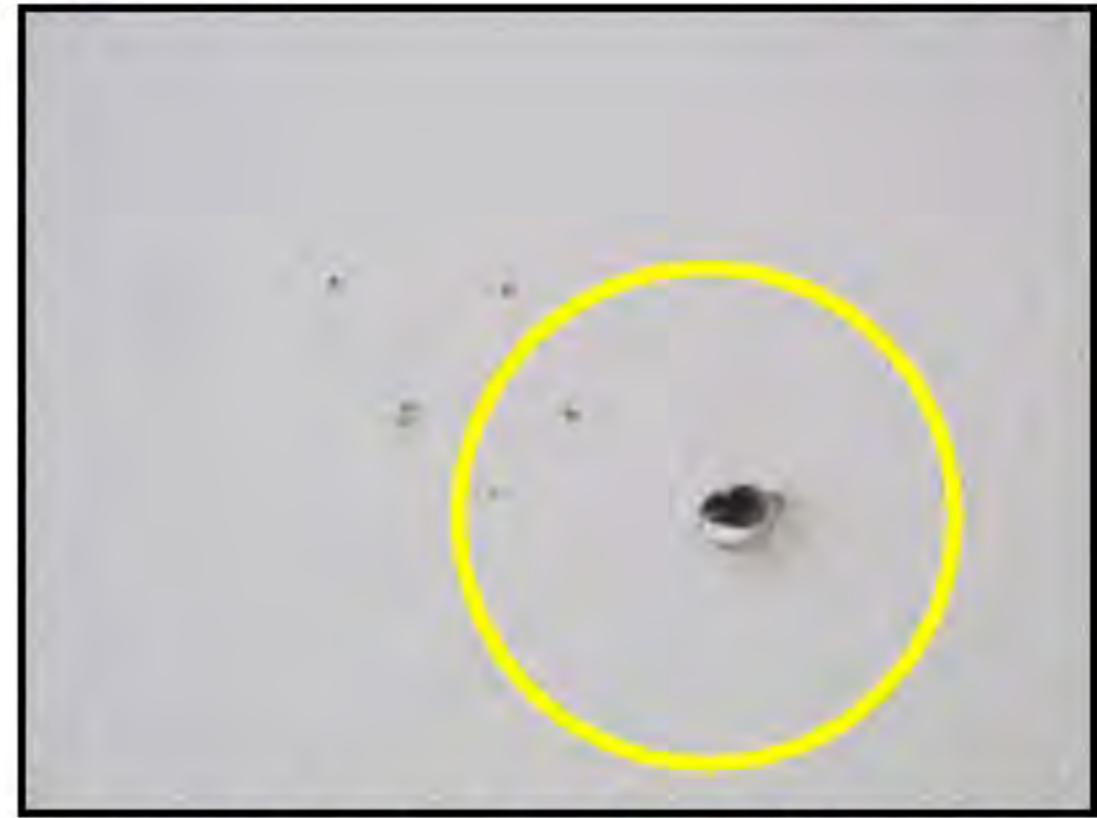
Minor Holes noted in Back Porch Ceiling
