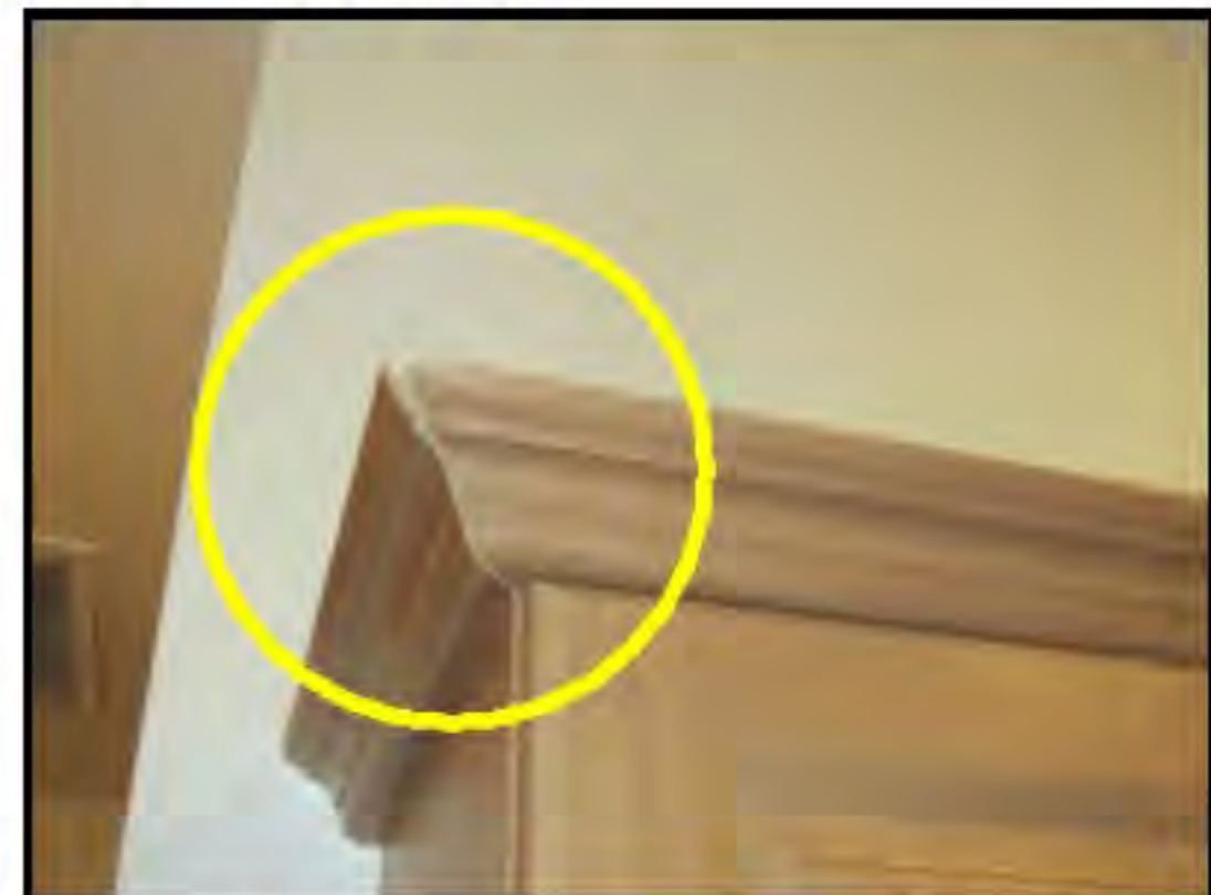
Crown molding loose in areas of Kitchen Cabinets
