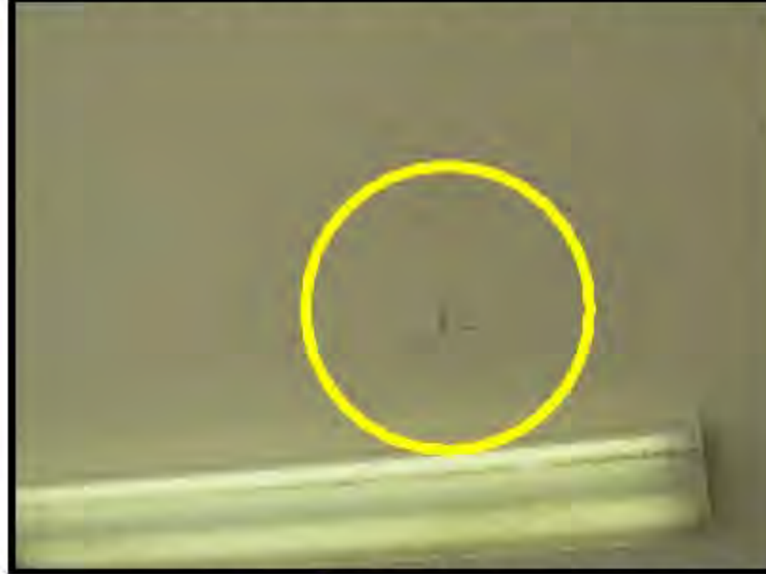
Minor crack/hole in ceiling
