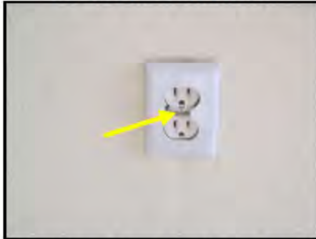
Outlet cover plate missing/broken in Front Bedroom
