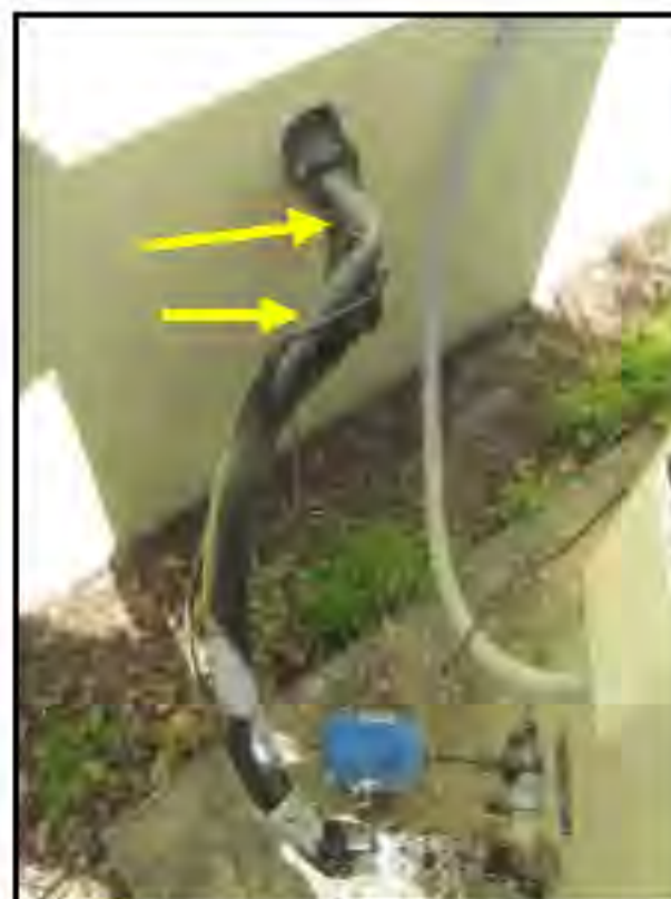
Missing insulation at A/C unit.
