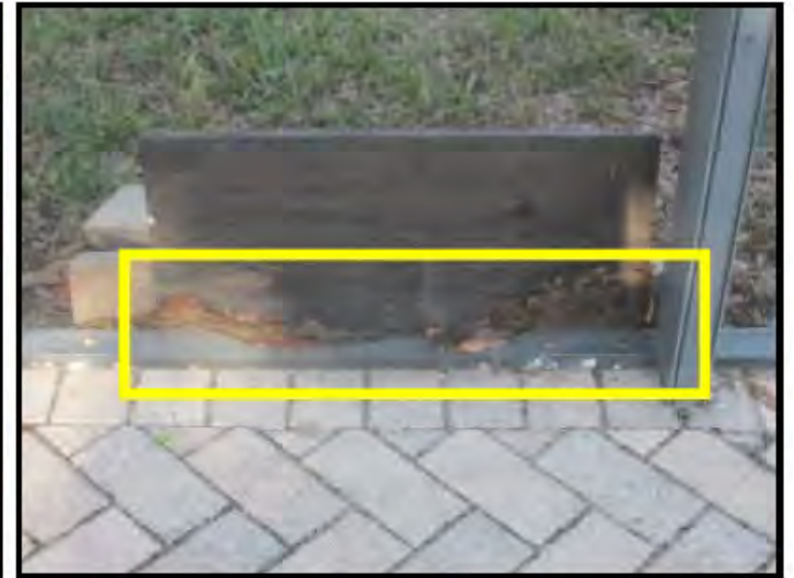
Screen loose/unattached in areas
