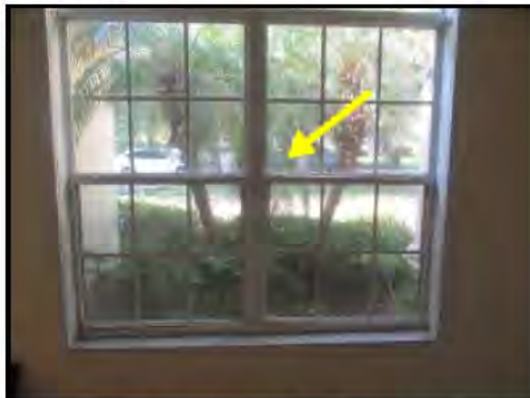
Front right window balance broken in Dining Area (window won't stay in the open position)
